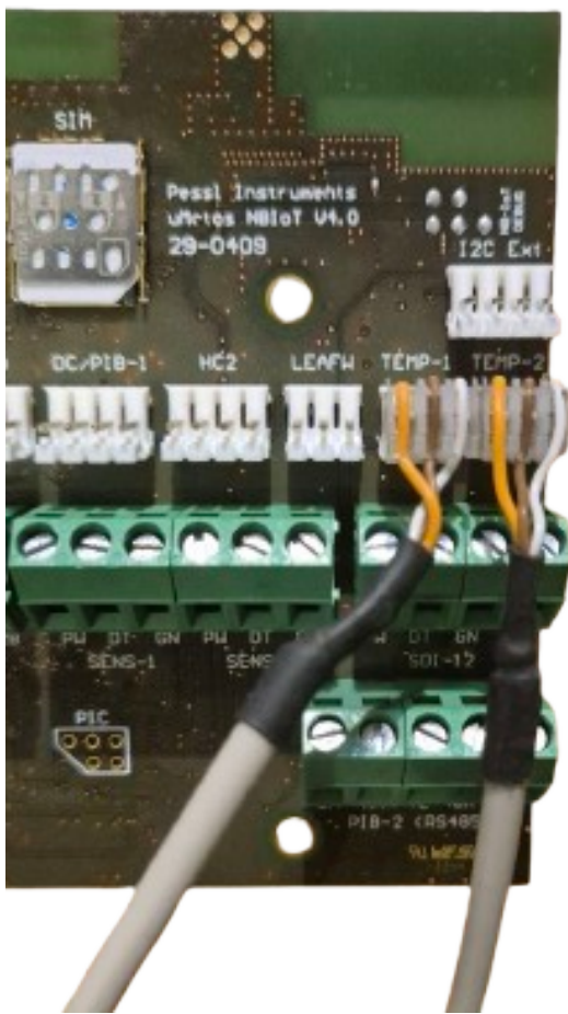
Photo of connect PI WM temperature Sensors on dedicated TEMP-1 and TEMP-2 inputs
