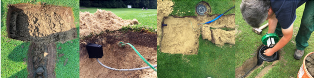
Cutting out the lawn tiles Laying the cable - inserting the sensors in the main turf root zone MiniMETOS SOIL installation: Preparation of the irrigation box for the data logger
